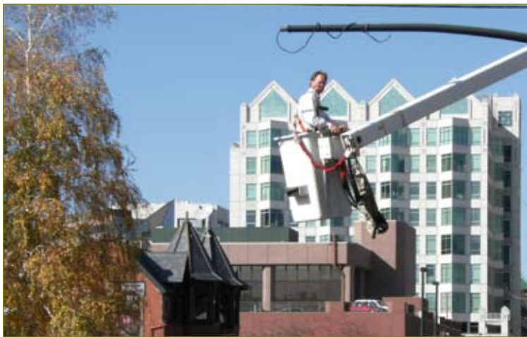
Changing traffic signals is just one of the steps in changing a one-way street back to two-way.
